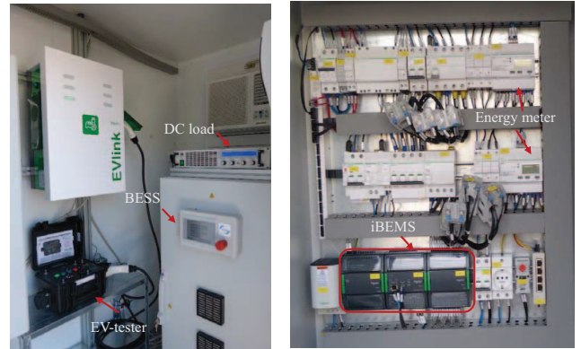
Fig. 2. From left to right, the pictures shows: the PV system with the EV-link, the EV tester, the BESS cabinet and the DC electronic load in the container. The rightmost picture displays the BEMS along with two energy meters.
