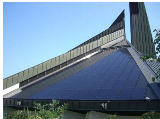
Figure 1: Roof-integrated PV system, Milland Church
