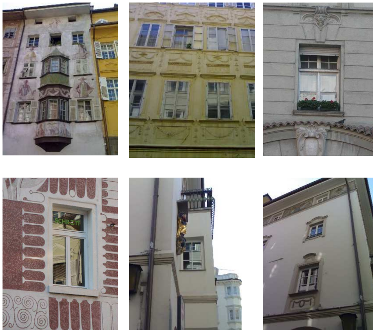
Figure 1-6: Originally, the wooden frames, impost and sash bars were very fragile and thin, possibly moulded (fig.1-3), while the optic of the typical replacements is much broader (simple application of the IV68 standard, fig.4-6).
