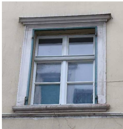
Figure 7-11: rotation of the frame cross section by 90 degrees (fig. 7-8) to achieve a smaller frame; separation of functions into two layers: “historic” window outside, integration of passive house window inside (fig. 9-10), last prototype installed in the Weigh House (fig. 11).
