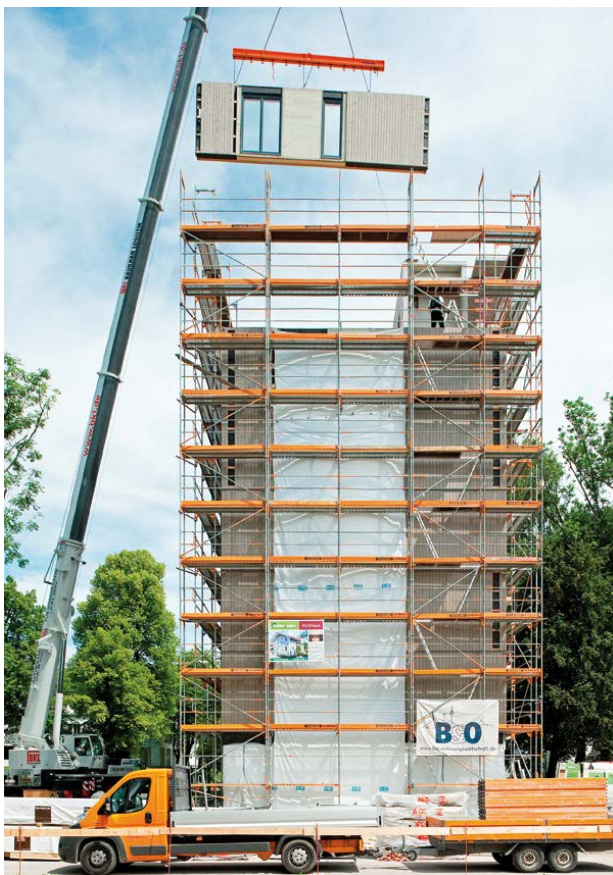
Fig. 9 Façade installation process for the Holz8 building in Bad Aibling (source: www.huber-sohn.de )
