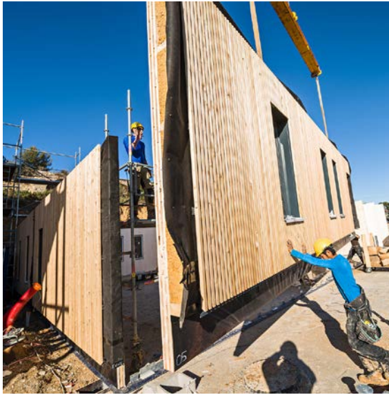
Fig. 11 Façade installation process for the Nexity Ywood «L’Ensoleillée II» building in Aix-en-Provence (source: ©Nexity, Yann Bouvier)
